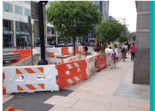
Figure 14. Longitudinal channelizers in Washington, D.C. (Image: Plastic Safety Systems Inc.)
