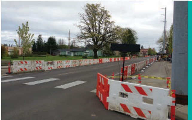
Figure 29. Longitudinal channelizers in Adair Village, Ore. (Image: Plastic Safety Systems Inc.)
