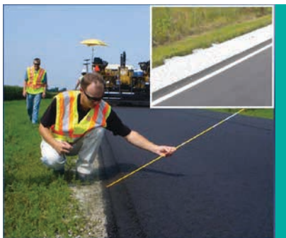
Figure 12. The Safety Edge SM (Image: FHWA)
