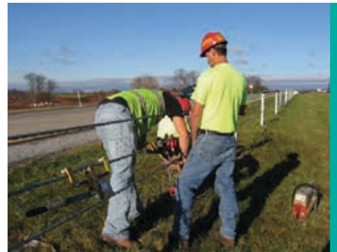
Figure 19. Sample of Cable Barrier System, Minnesota (Image: Mark J. Bloschock)
