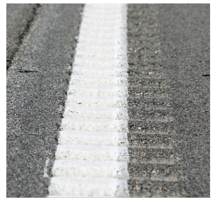
Example of an edge line rumble stripe.
